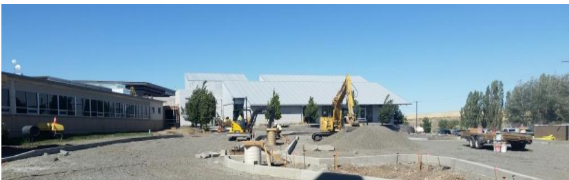
Below: The parking lot is being reworked for a safer approach to the school.
