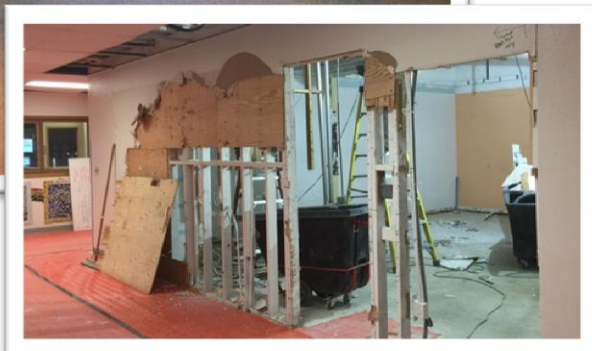
Above: A new student lounge is being constructed in the old workroom near the existing Jr./Sr. High Administrative Office.
