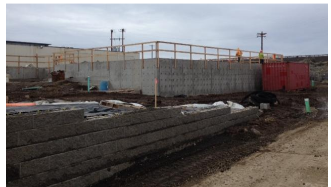
Left: First day serving in the new kitchen. Above: Phase II foundation and retaining wall.
